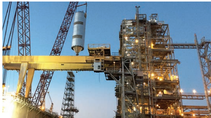
Maya II's coker drums represented part of over 6 million pounds safely lifted during a 12-day period of the turnaround.
